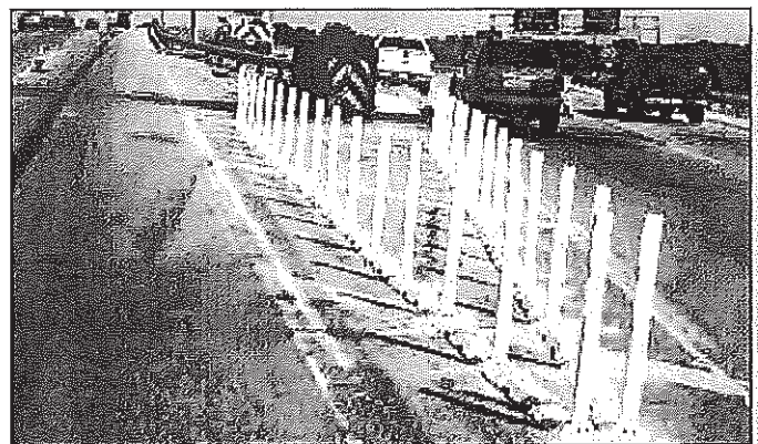
Impact attenuator protection
